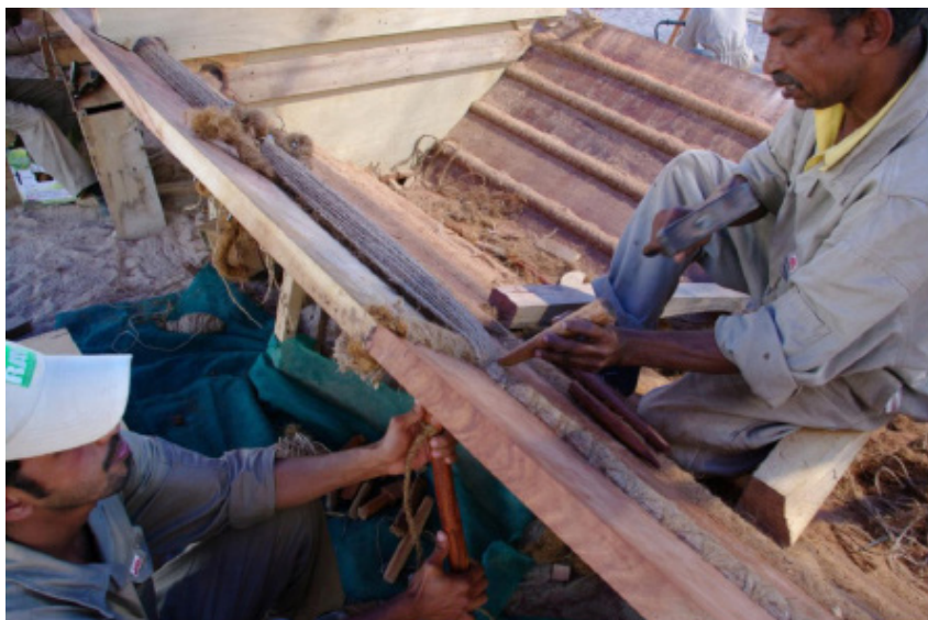
Figure 21. Caulking of the sewn ship Jewel of Muscat in Oman, photographed in 2009.
